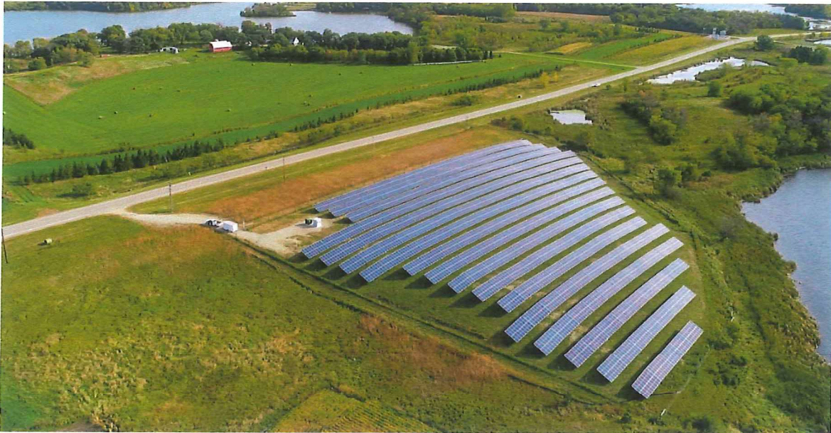
1MW CSG in Pope County
